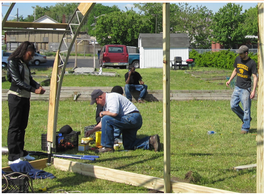
Constructing a hoop house located next to the Escher Street SRO in Trenton
